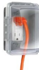
GFCI receptacle in weatherproof enclosure
